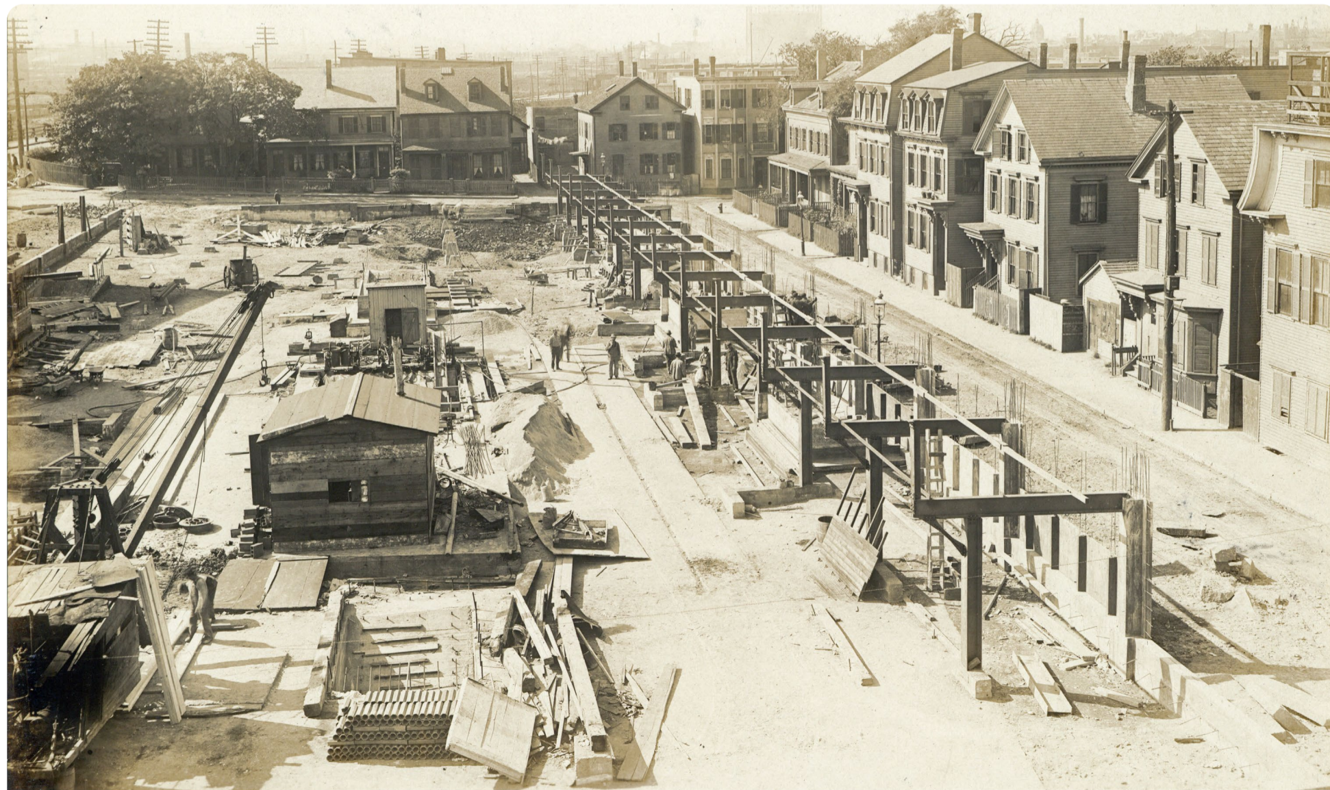
Dor. Tun. Sec. J. Birdseue view of Andrew Surface Station. looking W'ly. Oct. 2, 1917. #1550-D
