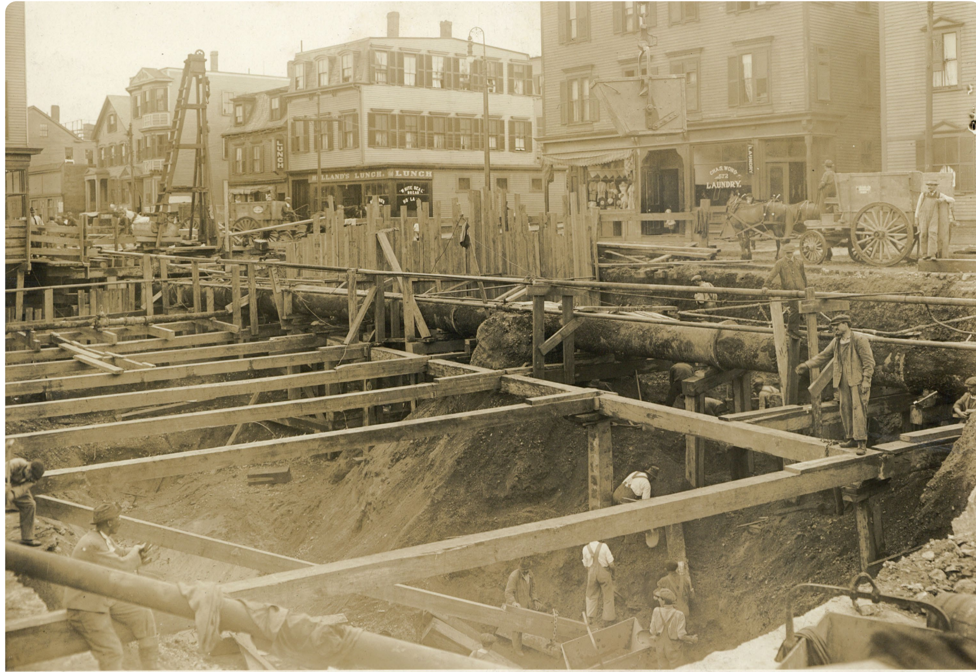
Dor. Tun. Sec. J, Excavation between Dexter Pl. and Dorch. Ave. June 20, 1916. #1154-D
